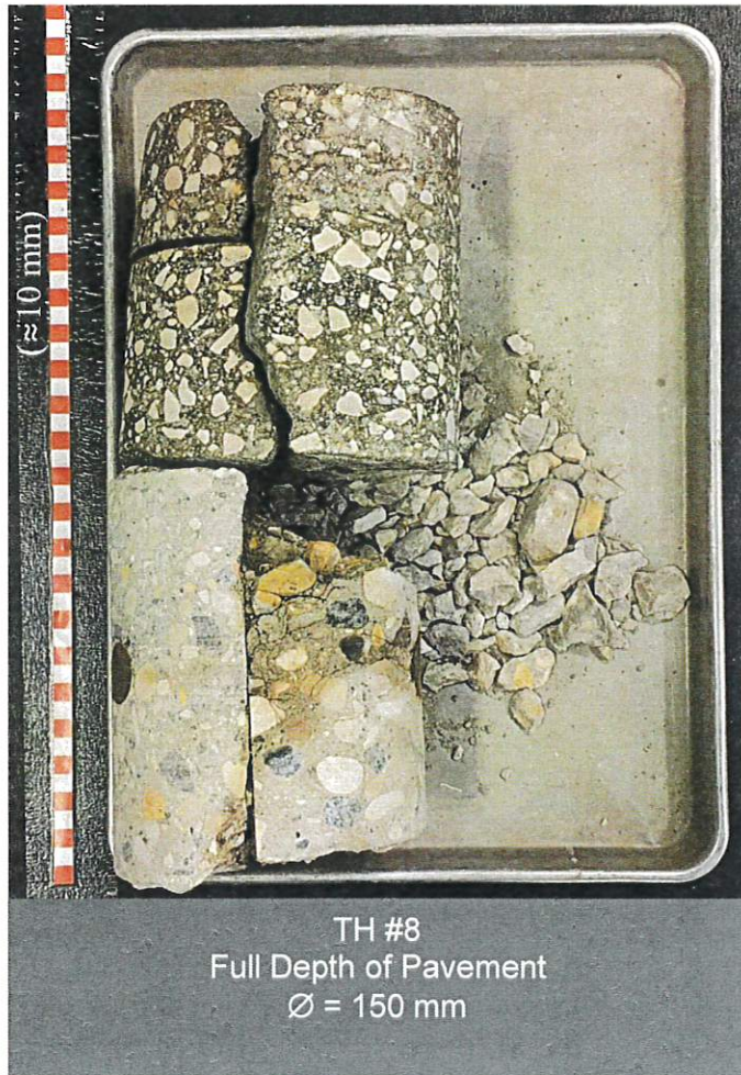
Photograph 30: Specimen from Bishop Grandin Boulevard, Eastbound Median Lane
