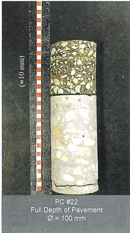
Photograph 22: Specimen from Bishop Grandin Boulevard, Eastbound Median Lane
