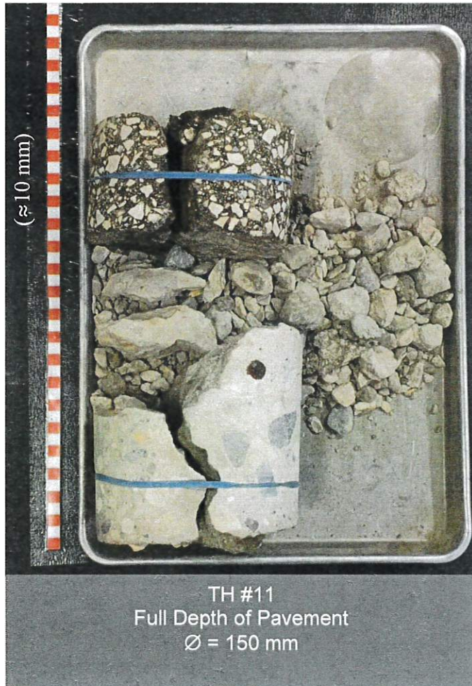
Photograph 33: Specimen from Bishop Grandin Boulevard, Eastbound Curb Lane
